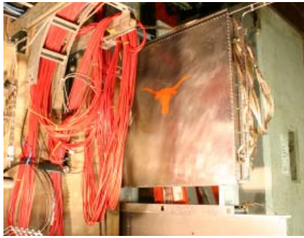
Figure 3: The hadron monitor during installation into the beam absorber. The monitor is installed on rails through a 2m(H)×15cm(W) slot in the concrete shielding.
