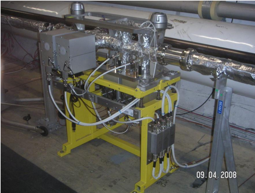
Wire-scanner location at 5R4
